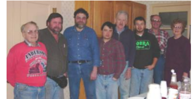
Lunch break at the home of Wesley and Esther Boese during the March 3 rd workday on gutting. From left: Pete Anderson, Bill Ongstad, Dan Fiesel, Kerry Ebel, Paul Gunderson, Jerome Gunderson, Wesley Boese, Esther Boese.
