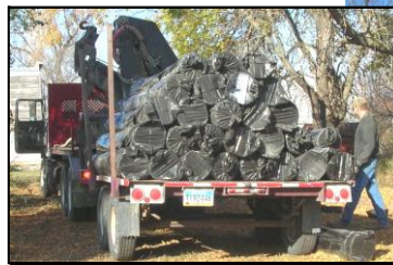
↑ Unloading drain file pipes and septic tank → to be installed on the north side of the house
